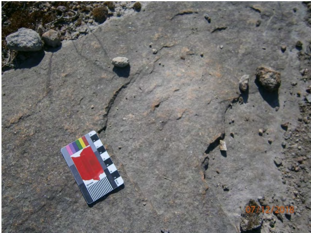
Figure 21: Machine damaged sandstone block in Stage One 7 December 2018
